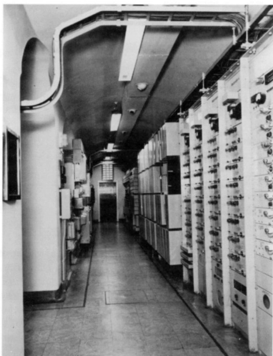
A view of the Apparatus Corridor. On the right, opposite the entrance to National Control are communications channels next to ATM metering panels. There is some switchgear on the left providing power to chargers and batteries located elsewhere.
