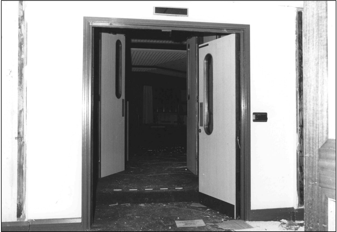
Plate 79: Control room (1F15), doorway from corridor 1F19 at NE corner showing swipe card, looking SE (photo 1/17).
