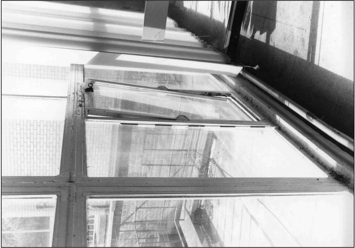
Plate 39: Former East Coast District Control Room (GF1), detail of window in W wall, looking NW (photo 4/13) (top to left).
