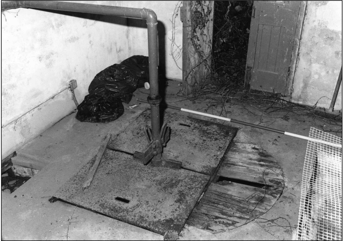
Plate 9: Interior of pump house, well, looking W (photo 9/11).
