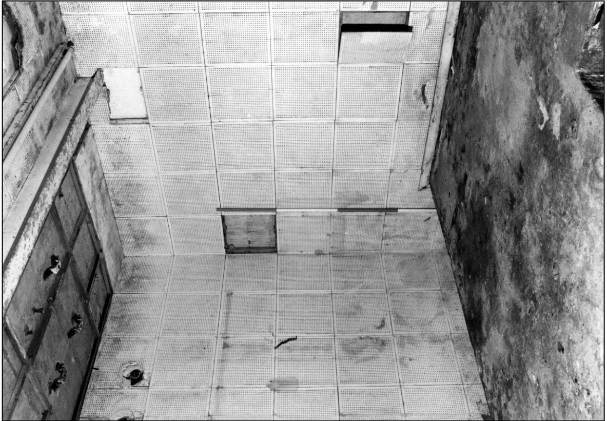
Plate 41: Generator Room (B5), looking S (photo 5/18) (top to left).
