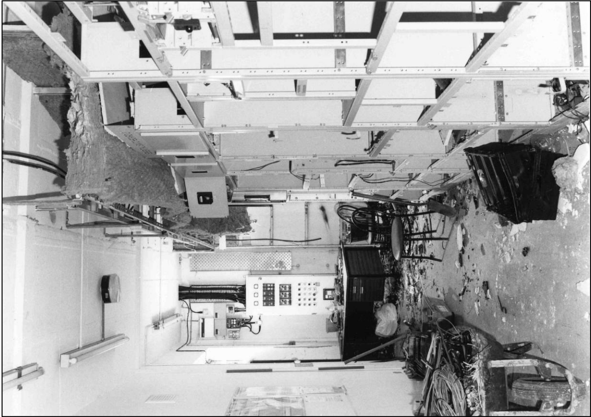
Plate 63: Essential Switchroom 2 (GF24), looking SW (photo 5/14) (top to left).
