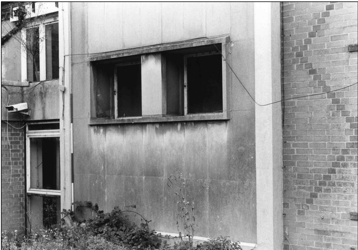
Plate 16: Control Centre complex, S end of E elevation, window detail, looking S (photo 7/9).
