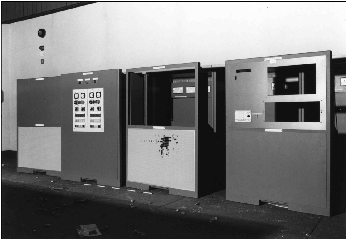
Plate 86: Control room (1F15), control panels to NE corner, looking NE (photo 1/16).
