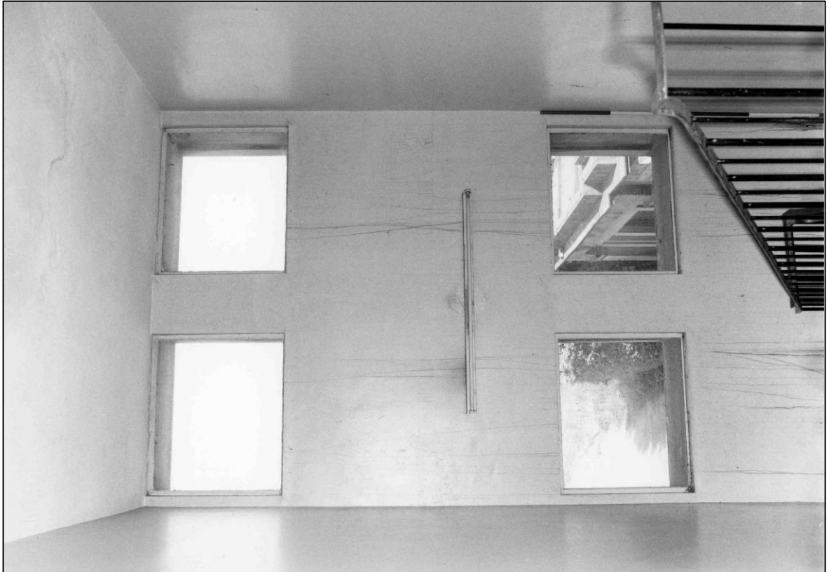
Plate 71: Staircase 1F4, windows to E wall, looking NE (photo 4/2) (top to left).
