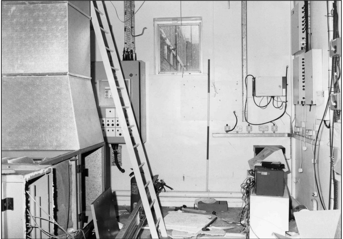
Plate 53: Air Conditioning and Security Room (GF7), looking NW (photo 4/11).
