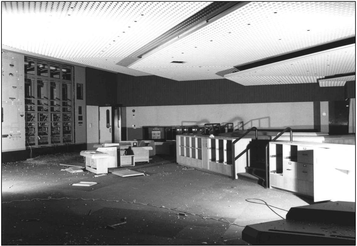
Plate 83: Control room (1F15), N end of mimic board and control desks, looking N (photo 1/12).
