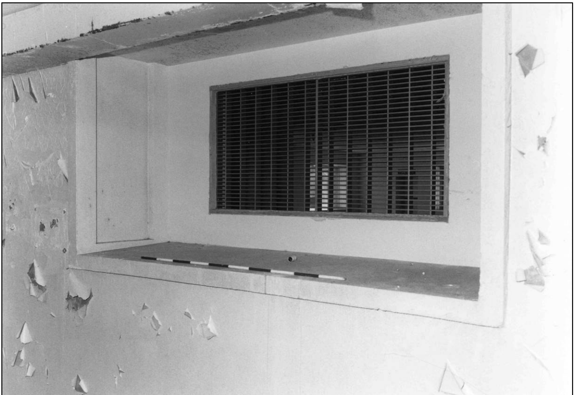
Plate 74: Corridor 1F6, blocked window at S end of W wall, looking S (photo 3/18).
