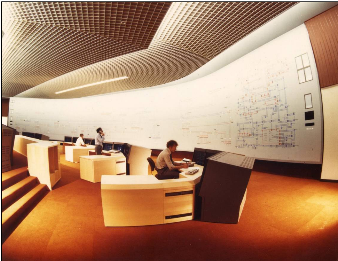
Top: Becca Hall and Control Centre, April 2008. Bottom: Control room (1F15) in use, showing mimic board in operation, late 1990s.
