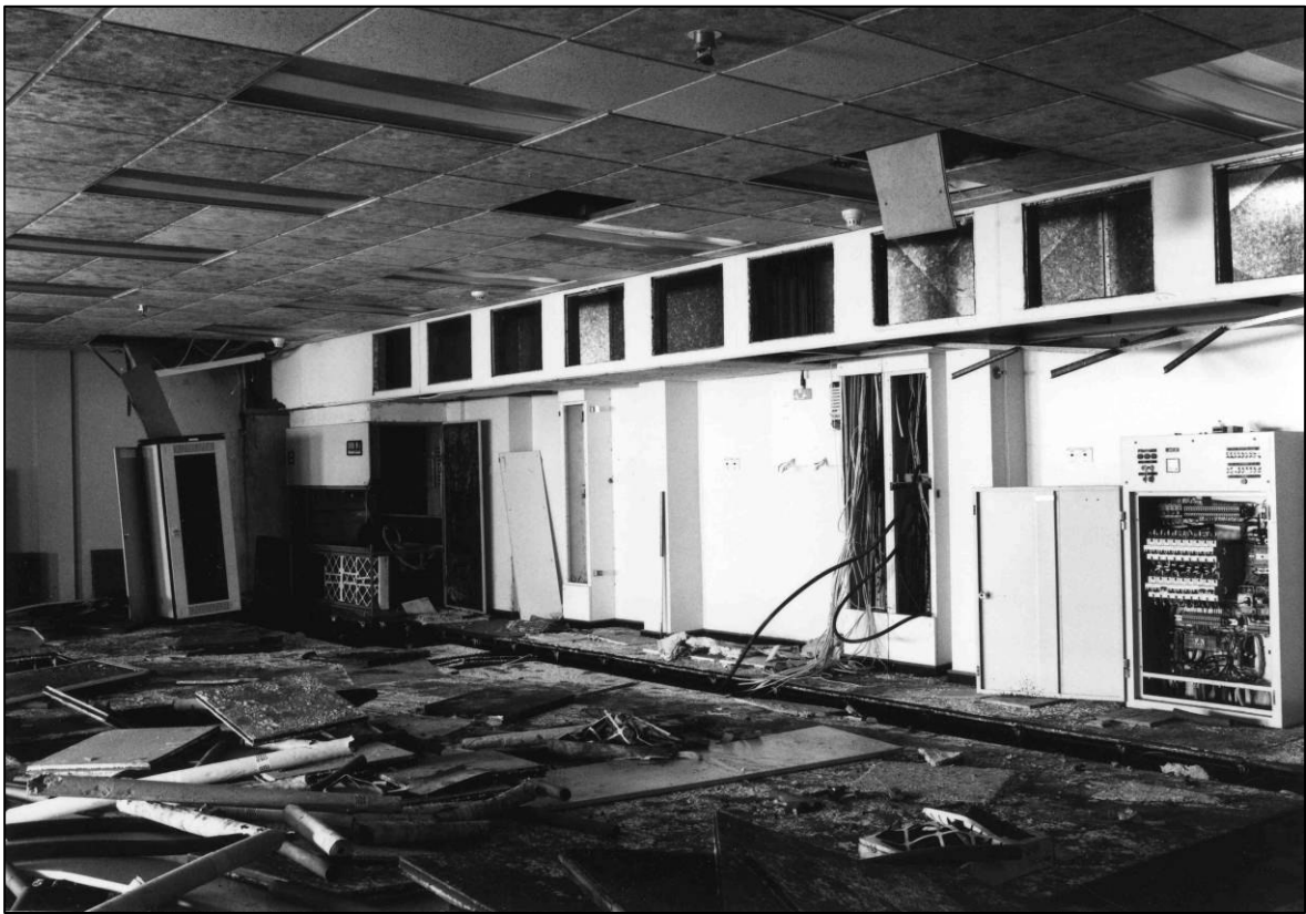
Plate 64: Apparatus Room 2A (GF30), looking E (photo 5/5).
