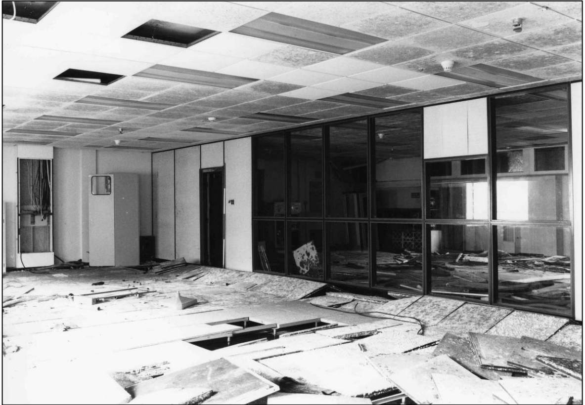
Plate 67: Apparatus Room 2B (GF31), looking E (photo 5/6).
