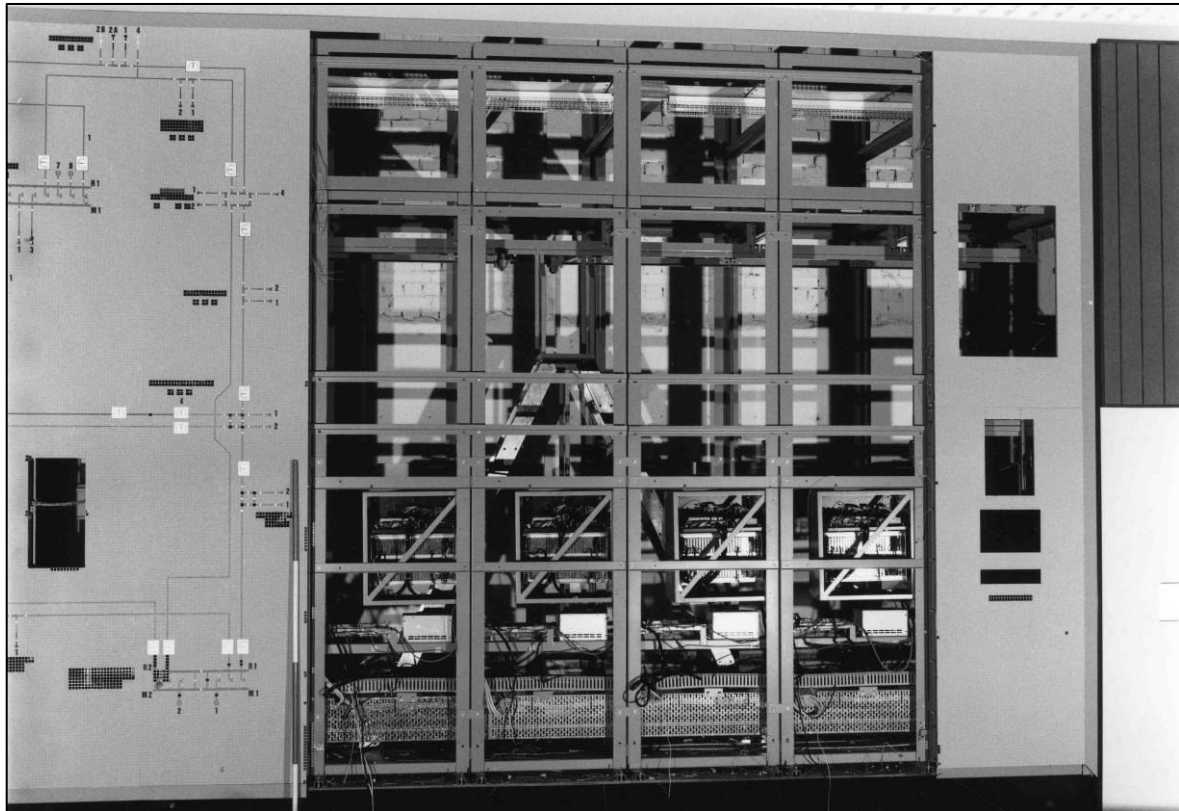
Plate 95: Control room (1F15), E end of mimic board, showing removed section, looking NW (photo 1/10).
