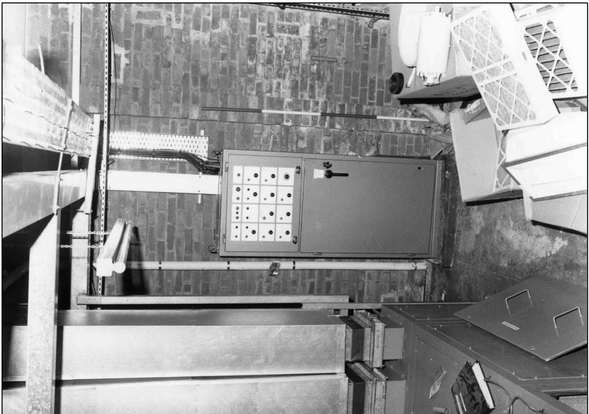
Plate 52: Air Conditioning Plant Room (GF9), looking SW (photo 4/16) (top to left).
